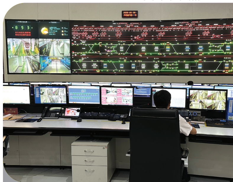
Luoyang Metro Dispatch Control Center
